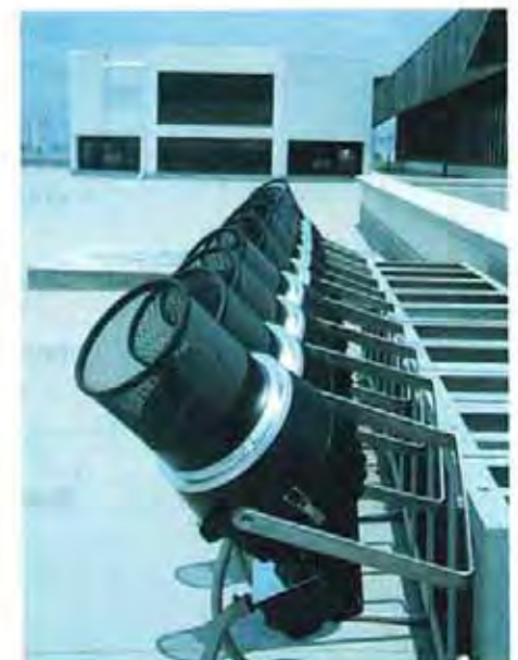
A row of narrow beam CSI floodlights used by Alan Russell to light up the main tower of the Putra Trade Centre.
